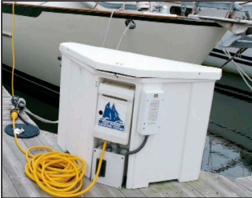
Figure 35-14 Typical utility cabinet found on marinas and boat docks
