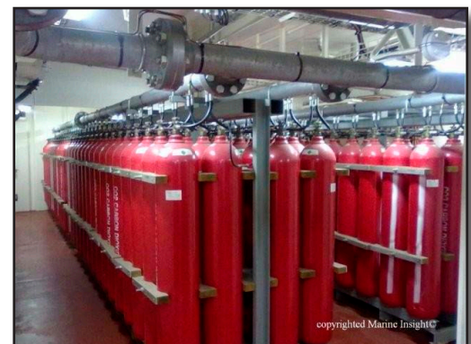
Figure 35-44 Many commercial vessels are equipped with carbon dioxide extinguishment systems similar to the one pictured here
